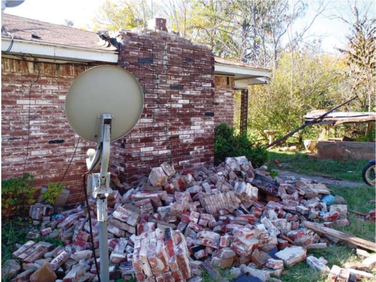
Earthquake damage in Oklahoma in 2011 linked to underground wastewater injection. Photo: Brian Sherrod/United States Geological Survey
